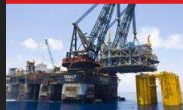
TENDON TENSION MONITORING
